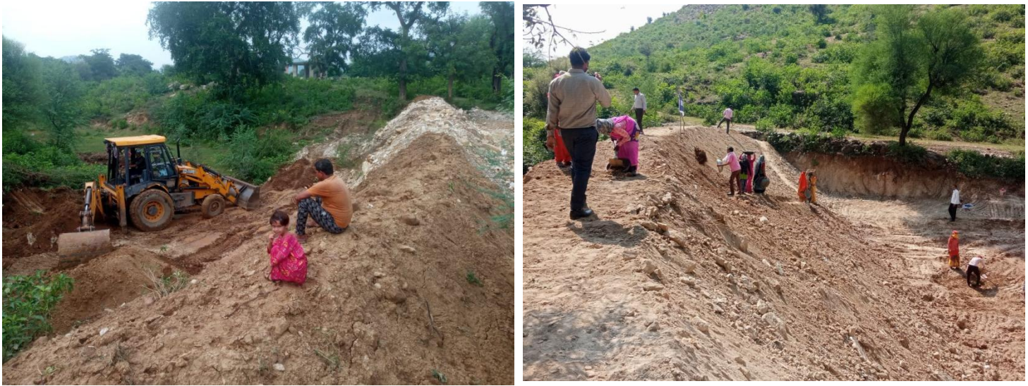
Fig 5,6 & 7 A traditional water body 'Johad' of 7926 m 3 (79,26,000 Litre) was created by community of 'Kakrali Rampura' village. Many migrant laborers who returned home because of COVID -19 became integral part of the work. Understanding the ground realities digging by hand was encouraged.
